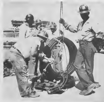
MECHANICAL-RIGGERS get lines ready as they prepare to unload the new bunkering tank. MECHANICAL-RIGGERS ta prepara linja pa haba e tanki pa bunker.
